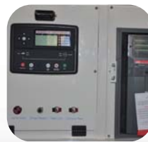
Control Panel & MCB
